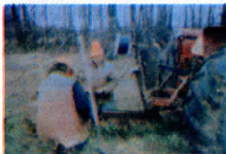
Subsoiler shank mounted on tractor 3-pt. is used to bury wire underground.
