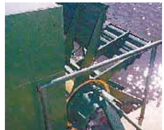
To make the paddle wheels he welded pairs of batts together side by side and welded them to steel support arms that he welded onto the wheels.
