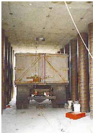
Twelve 18-in. dia. columns run along each wall of drive-through to support the silo floor, which is made of 15-in. thick reinforced concrete.
