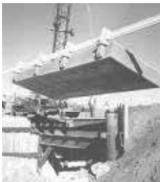
A crane was used to lower a 22-ft. long by 27-ft. wide fiberglass span - complete with guard rails - onto existing abutments.
