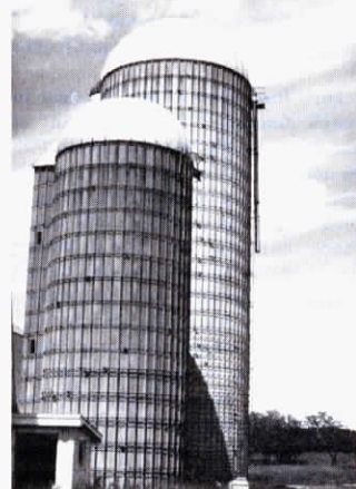
The results three days later of the straightening job provided by four experts from Madison Silo Co. Another company built the silo.
