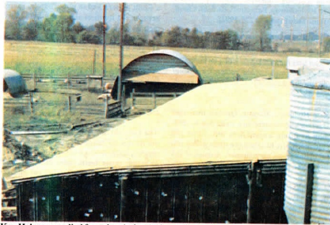
Ken Heberer applied foam insulation to the roof and sides of an open front hog building. "It stabilizes the interior environment," he says.
