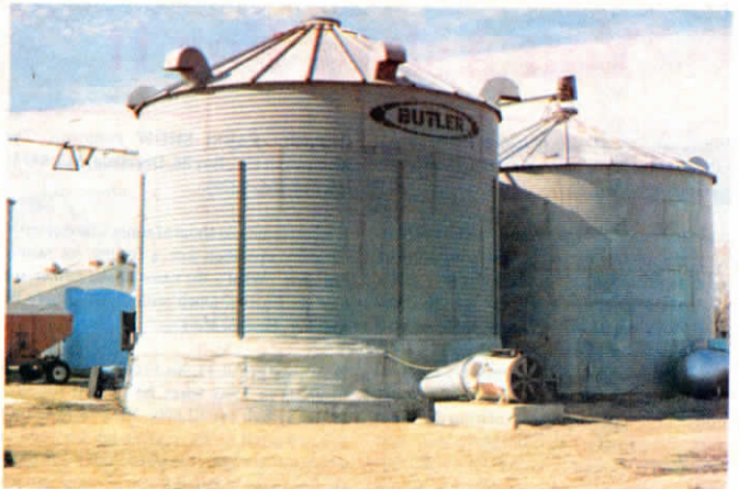
Nolan Harms says the 2-in. thick blanket of insulation around the bottom 4 to 5 ft. of his drying bin saves $1,000 a year on fuel.
