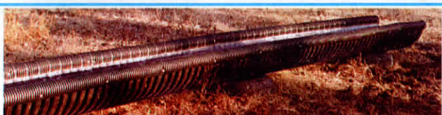
Pigg uses 20-ft. long sections of 24-in. dia. corrugated plastic culvert pipe, cutting the pipe in half lengthwise with a chainsaw.
