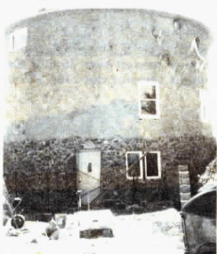
There's a 1-in. layer of foam insulation between the bin wall and the granite rock exterior.
