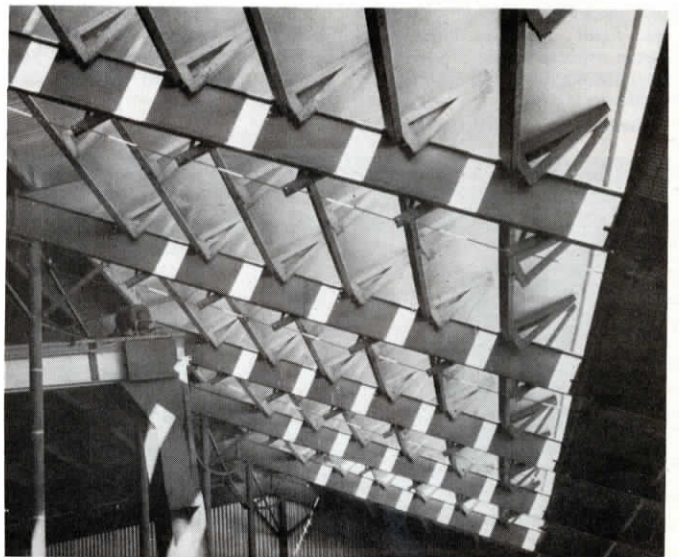
Jalousie-type louvers built into south-facing roof section open and close automatically to let sunshine in or keep rain and snow out.
