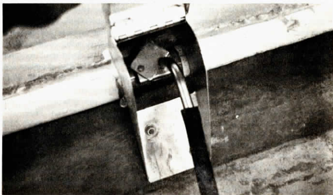
In this installation, the single line supplying the new-style milker was imbedded into the front curbing of the stanchions, thus eliminating any overhead pipes. Photo shows quick connect coupling at each stall.
