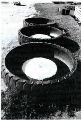
Kessler cuts off the top sidewalls of the tires, then attaches steel plate or concrete pads to the remaining tire bead to form the bottom of the tank.
