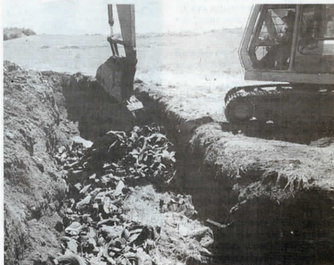
Ditches filled with chipped and shredded junk tires provide cheap protection against lagoon spills and leaks.
