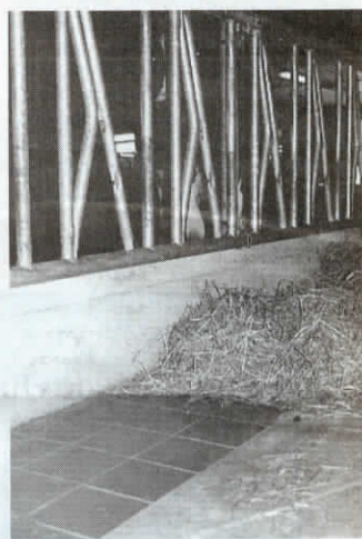
Ceramic tiles installed in mangers are easy to clean and wear like iron.
