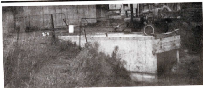
Manure flows from barn to lagoon via this 50-ft. long, non-sloping concrete culvert.
