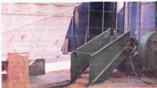
For grain, KIS conveyor feeder and recessed chase are covered with planking so truck can drive over for unloading.
