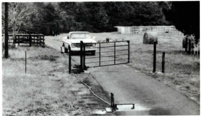
"Triggers" on either side of gate activate opener as vehicle drives through.
