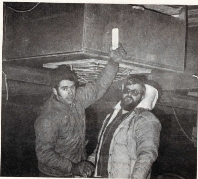
Darrel Thurnbeck, left, and Tom Rauenhorst check Beaver heat exchanger recently installed in Thurnbeck's turkey barn. During winter months, outgoing warm foul air is used to reduce temperature of incoming cold air about 23°F.
