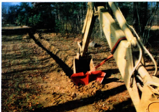
Trencher pulls through the ground like a plow to create smooth, 24-in. deep V-shaped trench.
