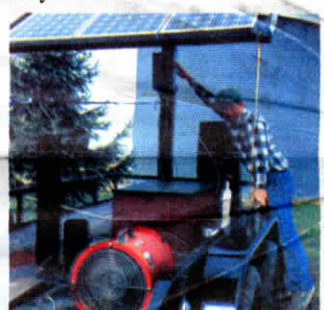
Switchbox mounted on pole is used to start motor and pump.
