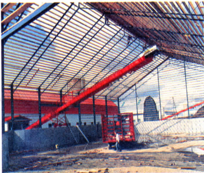
The 80 ft. wide, 100 ft. long, and 30 ft. high building has cement floor surrounded by 8-ft. high retaining wall.
