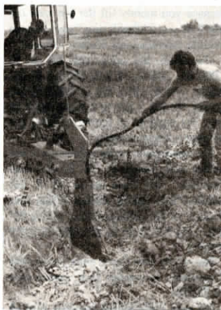
A field can be tiled every 15 ft. with 1 1/2-in. plastic tile for the same cost as conventional 4-in. tile at 50 ft., says Persall.
