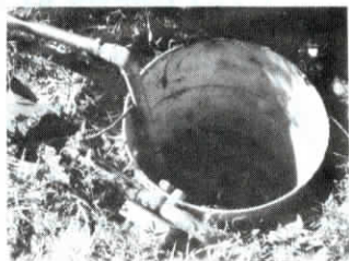
Partially buried 55-gal. drum receives water from the 1 1/2-in. collector pipes.
