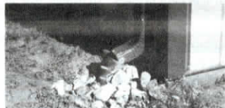
A funnel attached to a downspout directs rainwater into a buried plastic pipe.
