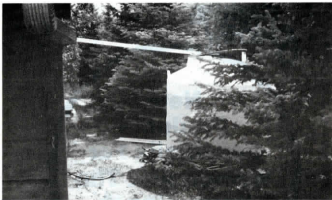
The 1,500 gal. tank receives pumped water from a 3,600 sq. ft. metal building and also direct runoff from a nearby garage.
